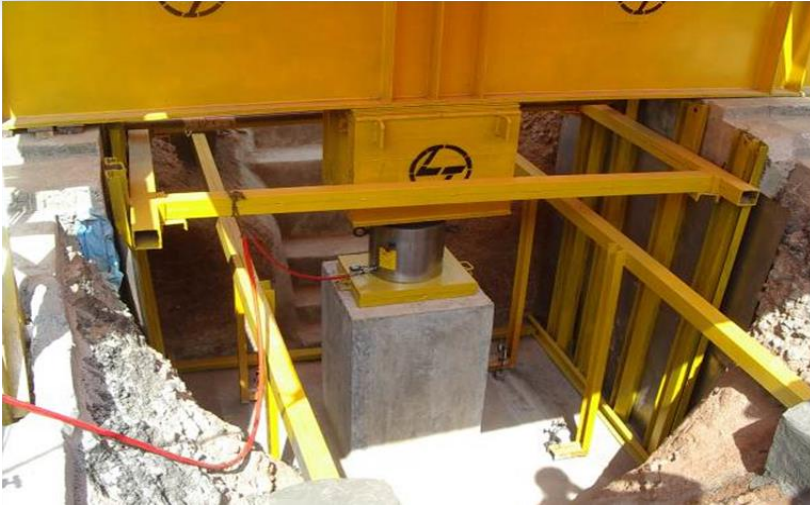
Utility probing being done to verify presence of any utilities at the site
