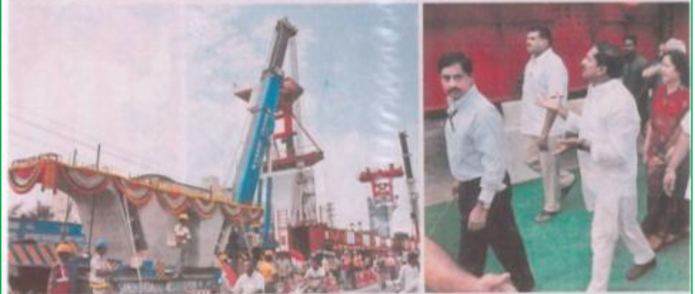
ON THE TRACK: The first girder of Hyderabad Metro Rail Project on overpass, between Uppal-Habsiguda was launched by Chief Minister N. Kiran Kumar Reddy on Sunday. - PHOTOS: G. KRISHNASWAMY
