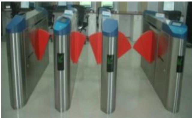
Automatic Fare Collection gates
